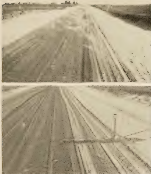
FIGURE 5.—A, SAND DRIFTING ACROSS A CUT-BACK SECTION. THE WIND WAS BLOWING TOWARD THE CAMERA AND AT A SLIGHT ANGLE TO THE CENTERLINE OF THE ROAD. B, DRIFTED SAND ON A LOOSE, ROAD-OIL SECTION. THE SPADE MARKS THE RIGHT EDGE OF THE BITUMINOUS MAT.
